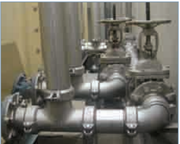
Domestic Water Service
