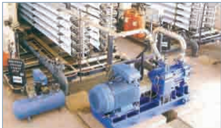
Reverse osmosis plant
