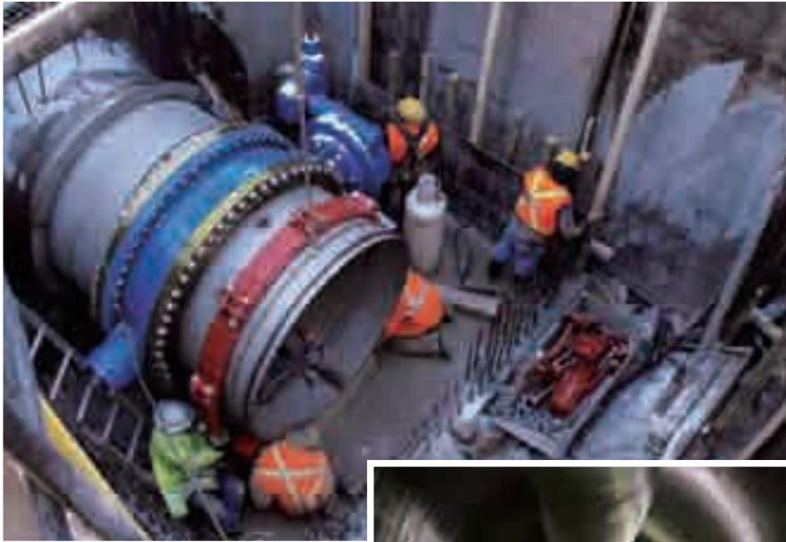
72" (1800mm) Model R-88 couplings used in a domestic water treatment plant, Ontario, Canada
