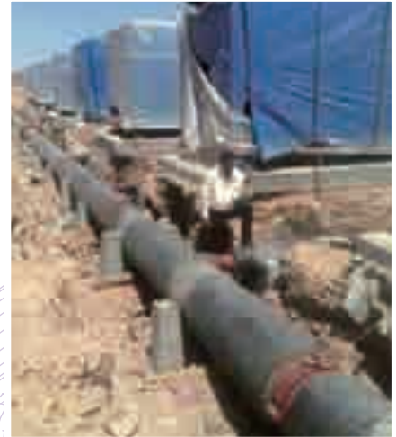
36" (900mm) Model R-88 couplings used in an HVAC chilled water line for a major university, Saudi Arabic
