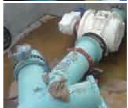
48" (1,200mm) Model R-88 couplings used in a water treatment plant, Quarry, Utah, USA
