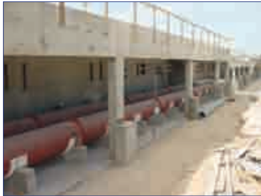
30" 7707L couplings on a chill water system
